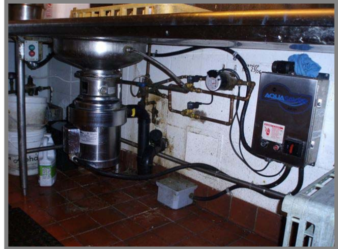
Garburator with water meter and flow control.
